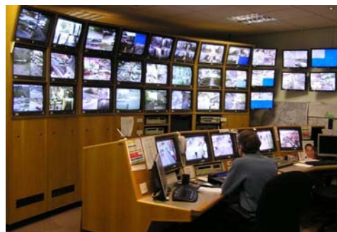
Figure 6: CCTV Control Room
